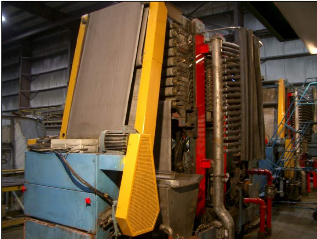
Figure 17-9 Mount Polley Larox Filter used to Dewater Concentrate
