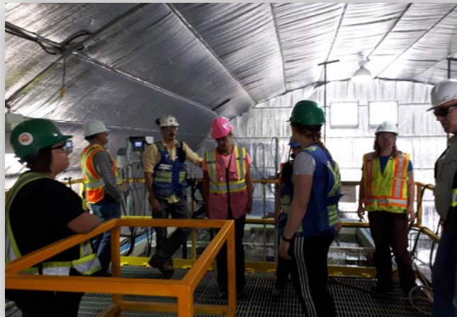
Tour group with additional MPMC environmental field staff explaining the different components of the WTP on top of the cells at the plant.
