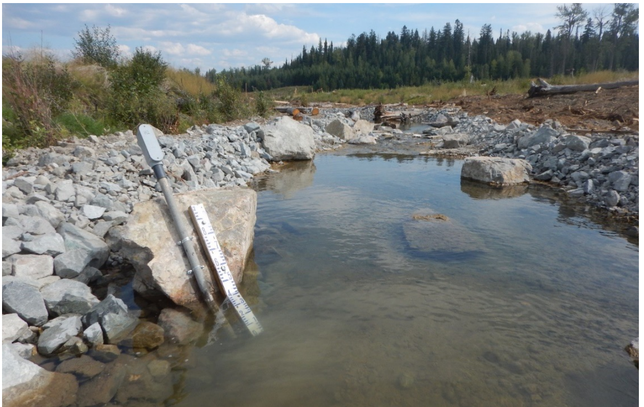
Figure 2 Newly installed H2 hydrological monitoring station. The original station was removed to facilitate instream remediation
