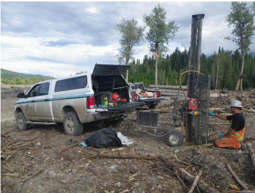
Photograph 2: Drilling MW16-09 in the Lower Hazeltine Floodplain Using the Truck-Mounted Solid Stem Auger Drill Rig
