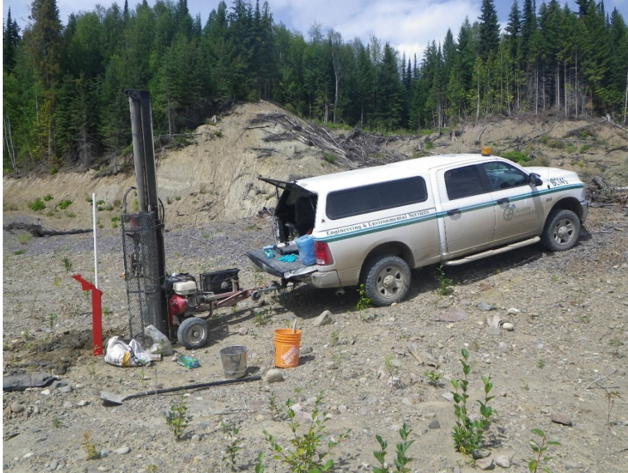
Figure 2: Typical drilling set-up, Including Installation of a Monitoring Well at the Mine
