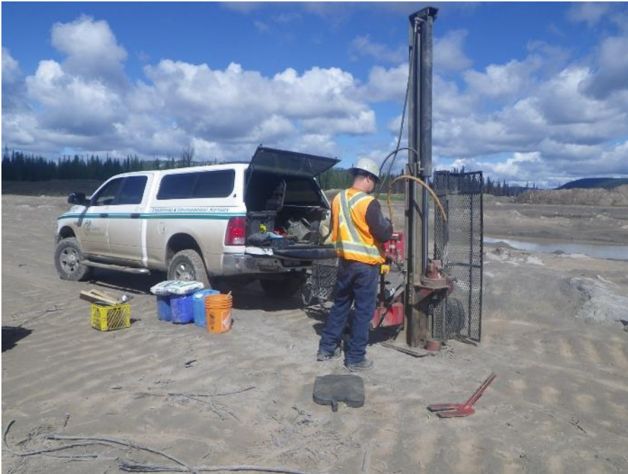
Photograph 1: Drilling MW16-01 in the Polley Plug Flats Using the Truck-Mounted Solid Stem Auger Drill Rig
